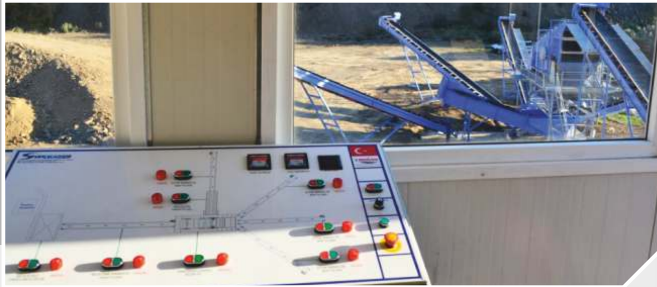
FIXED PLANT CONTROL PANEL
