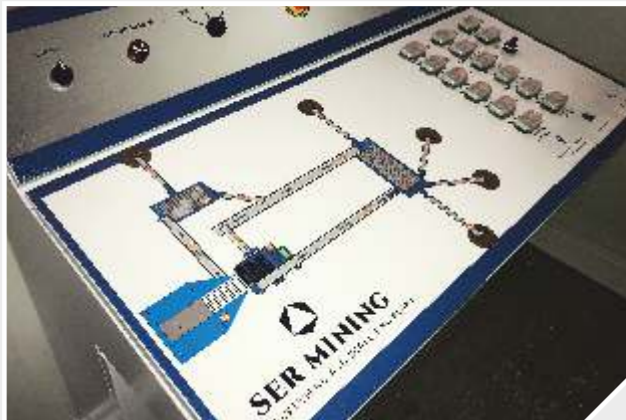
FIXED PLANT CONTROL PANEL
