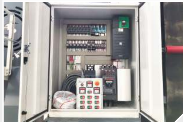
MOBILE PLANT CONTROL PANEL
